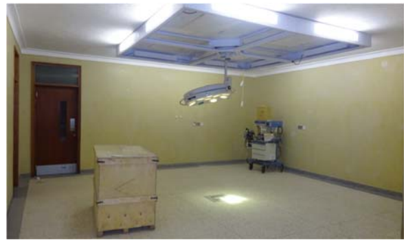
Operating Room Light Installed
